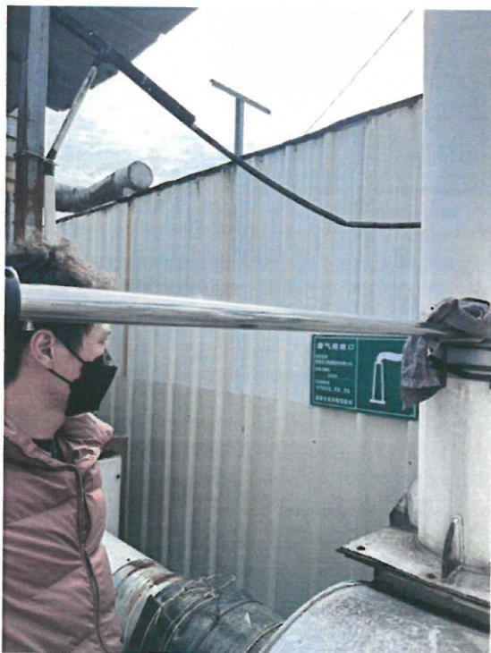
污水处理废气排气筒出口(FQPK-0006)G6
